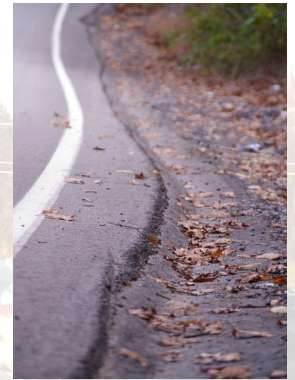
The pavement edge drop off in this photo is an example of a potential safety issue that could be identified in a RSA or an ISRSR.
